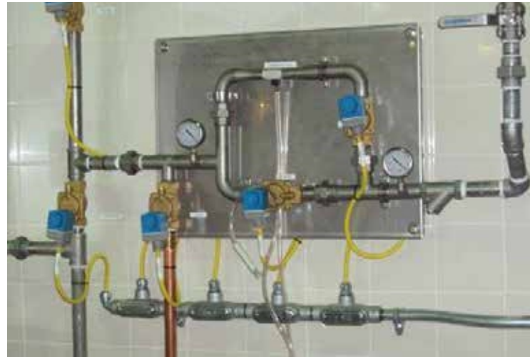
Automatic cleaning system.
