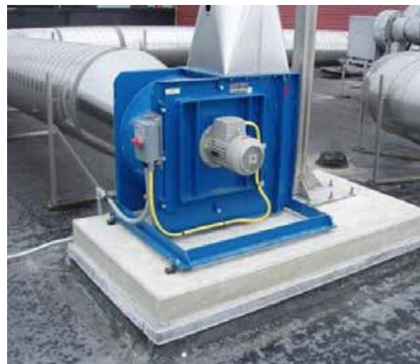
Fan placed on the roof.
