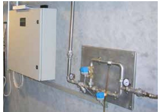
Control Board Automatic CIP cleaning unit.
