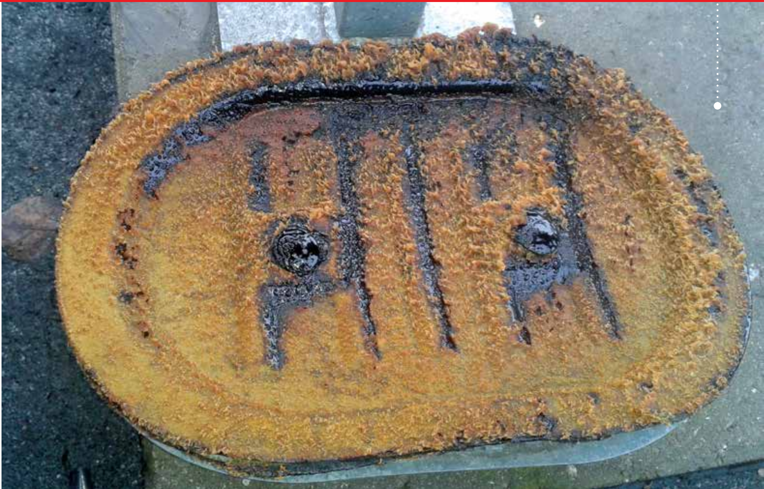
Inspection Hatch without JIMCO Technology - Not cleaned for 12 months
