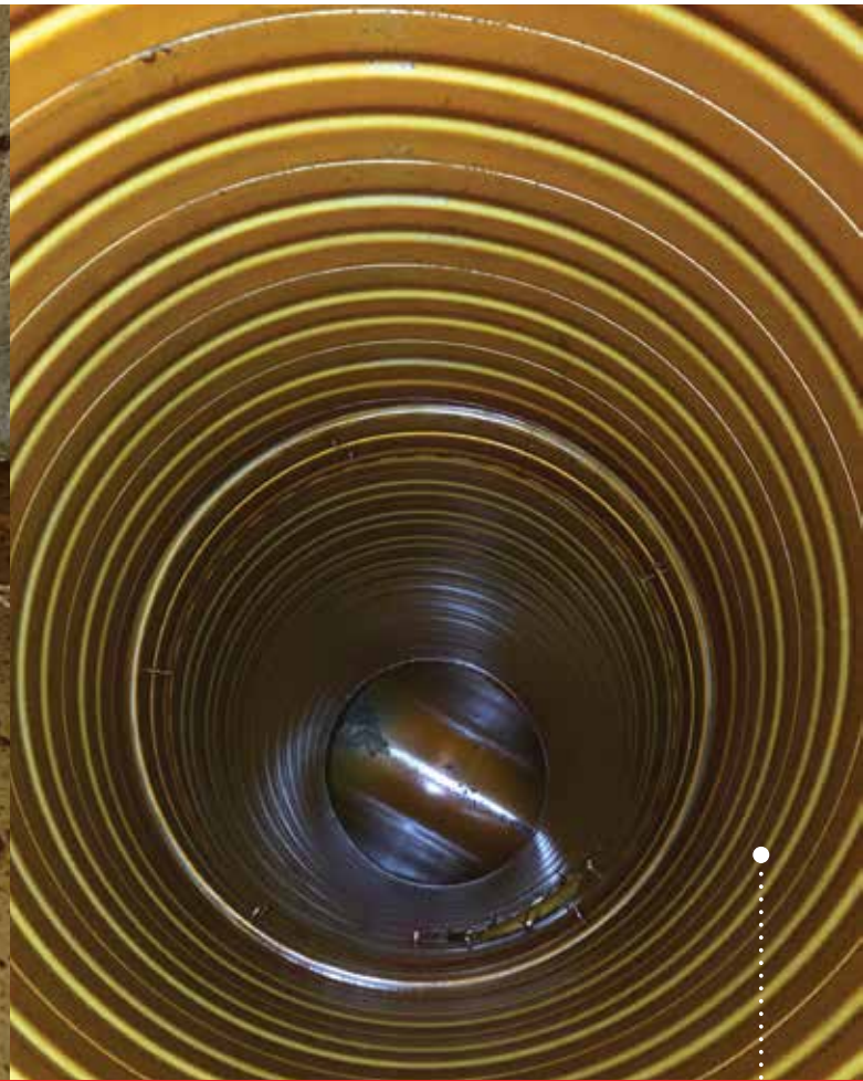
Fryer duct with JIMCO Technology - Not cleaned for 60 months
